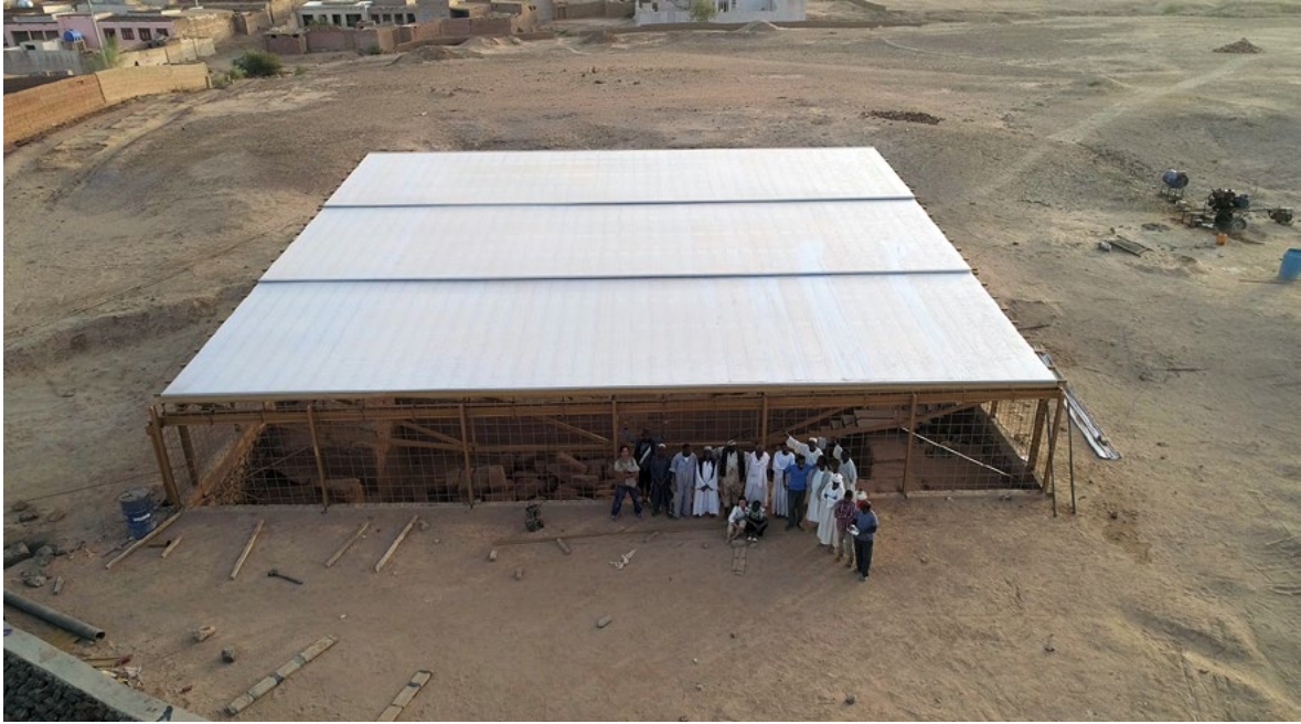
Figure 5. Completed cover over the funerary temple at El-Kurru with building crew. Drone photo: Sami Elamin, National Corporation for Antiquities and Museums (Sudan), 2020.
